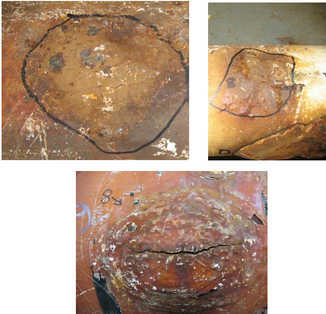
Figure A1-1: Examples of early stage external corrosion which has formed blisters underneath the coating. Note the cracks in the coating in the upper left and lower examples.
