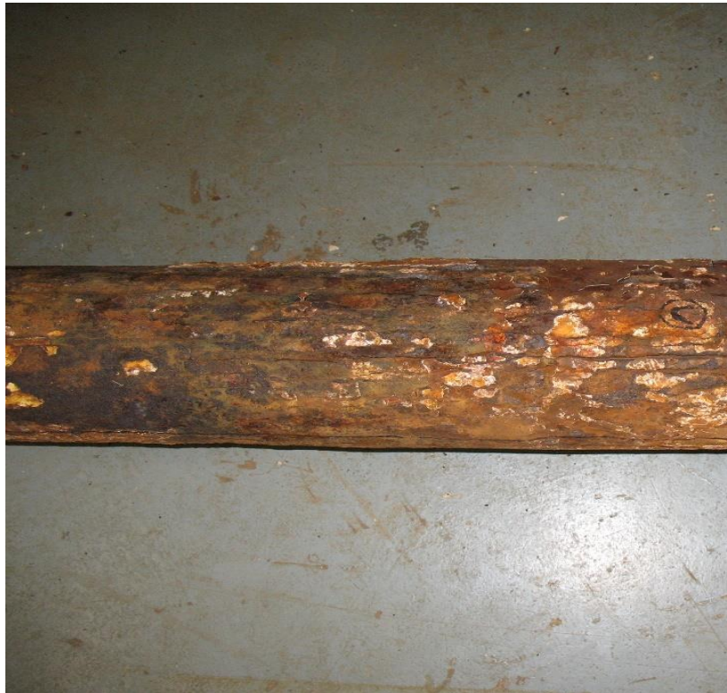
Figure A1-4: Example of widely distributed external corrosion with partial loss of coating
